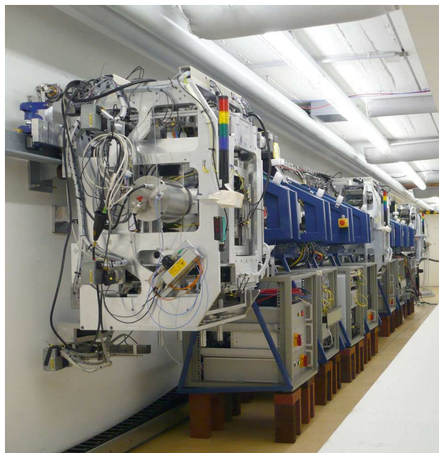
Figure 1: The prototype RTRS after commissioning in the DESY test tunnel (Jan. 2008). The electronics crates in the service cars have temporarily been supported by metal bricks during an analysis of vibration sources.
